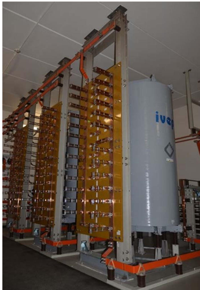
Fig. 2: High voltage part of the Laboratory of high currents
