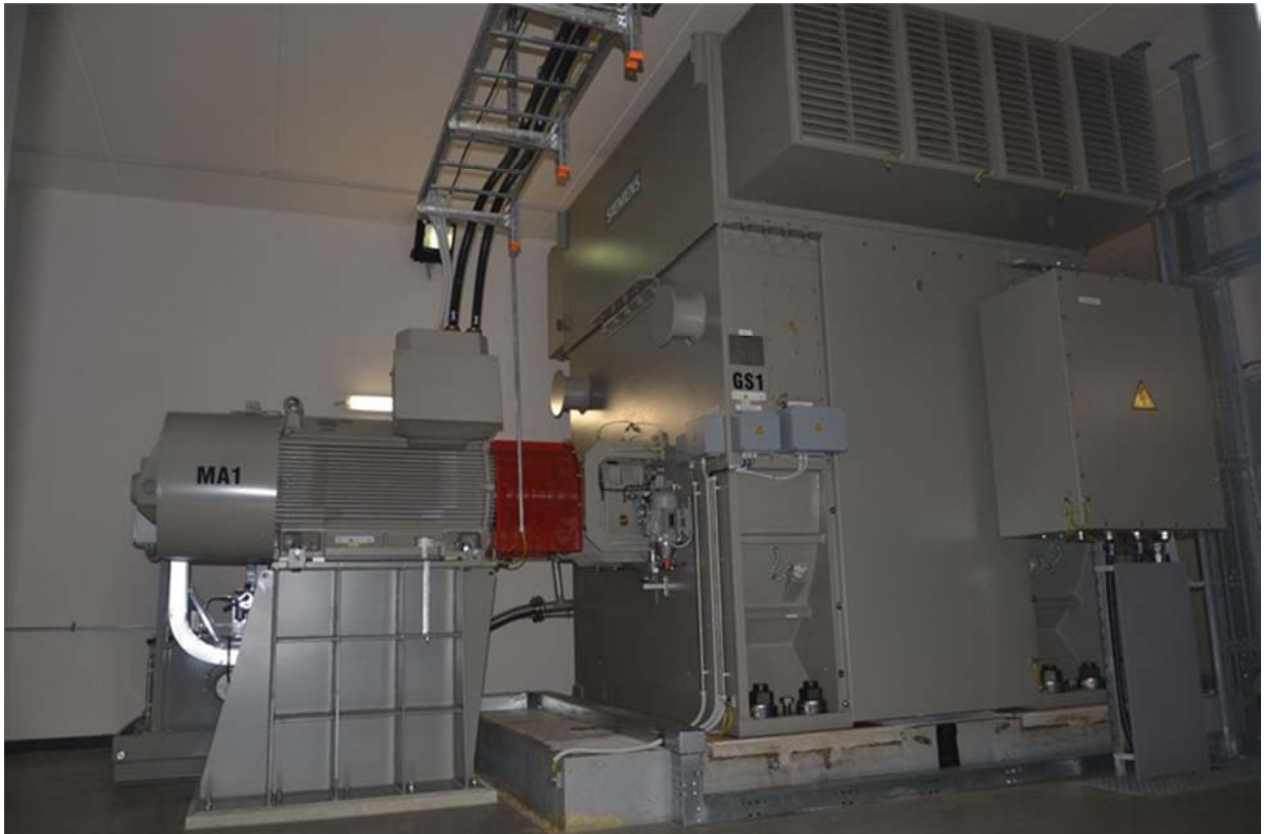
Fig.3: Generator of the Laboratory of high currents
